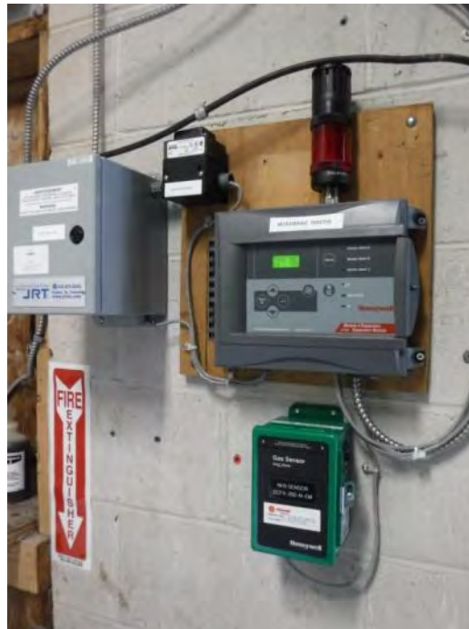
M3: Refrigeration Monitoring System (installed in 2018)
