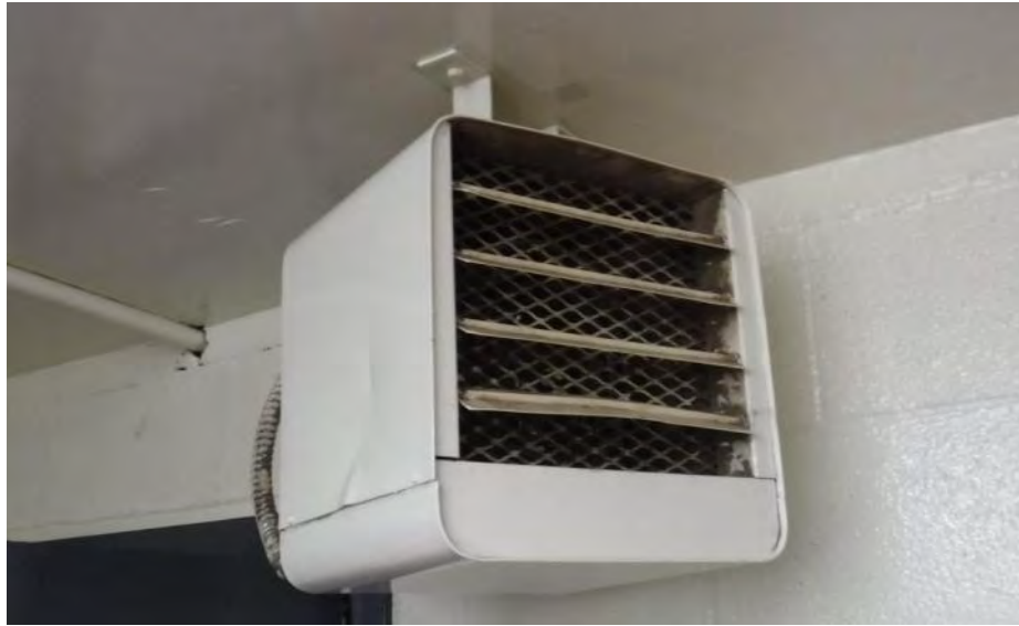
M16: Dressing Room – Electric Unit Heater
