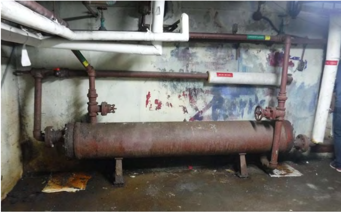
M14: Mech. Room – Ice Surface Heat Exchanger for converting to in-Floor heating with Boiler Water
