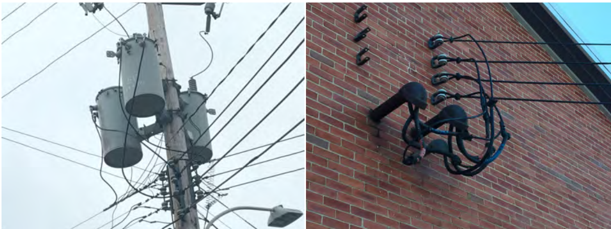
E6: 600/208-120VAC 3 phase 4 wire building electrical entrance
