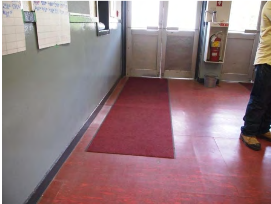
A5: Foyer. Poor door seal, non-barrier-free ticket booth
