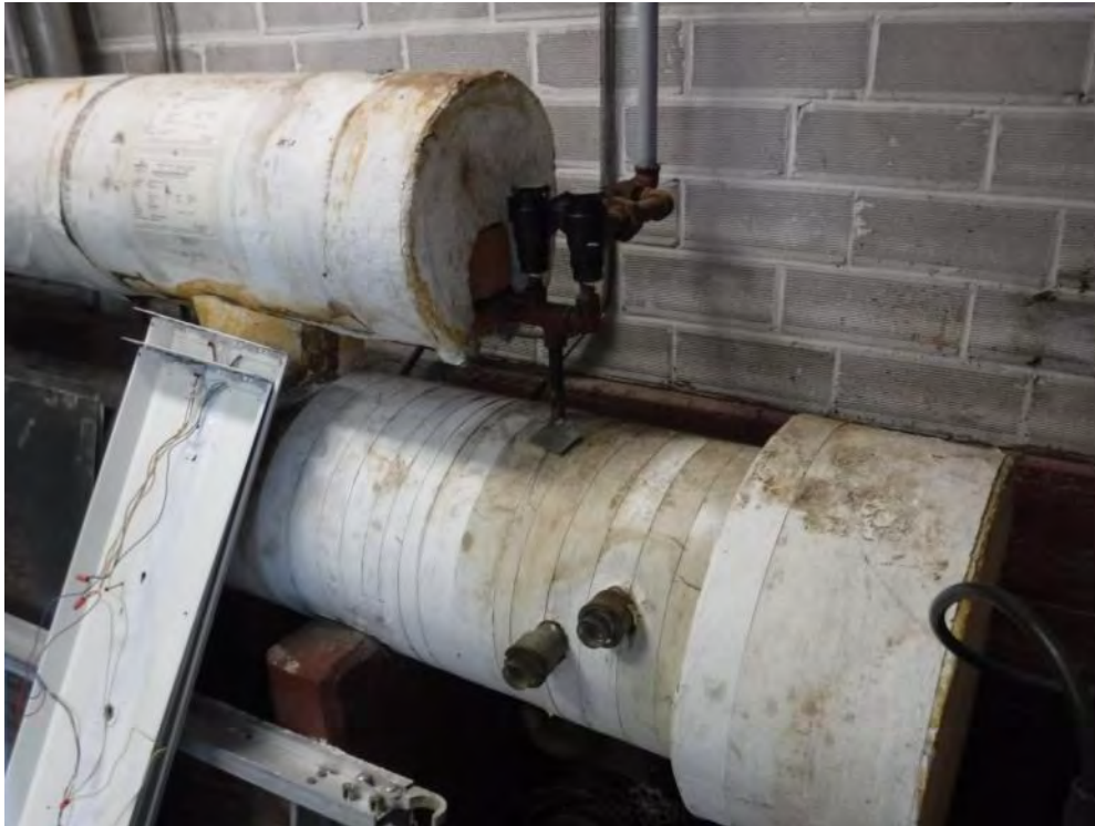
M5: Refrigeration Plant - Chiller with staging / light fixture leaning on equipment (installed in 1994)
