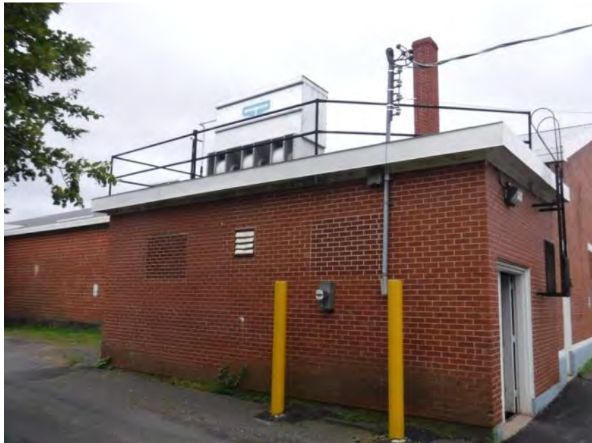
M2: Refrigeration Plant Gravity Backdraft damper damaged
