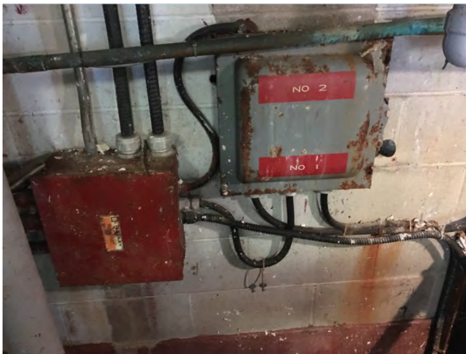
E2: Town Water line running on top of a 3-phase 600VAC manual Transfer Switch
