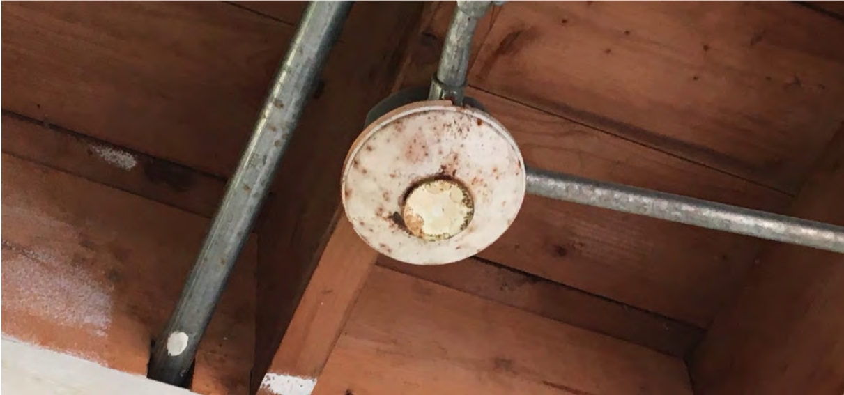
E14: Smoke detectors are well past 10 year replacement recommendation
