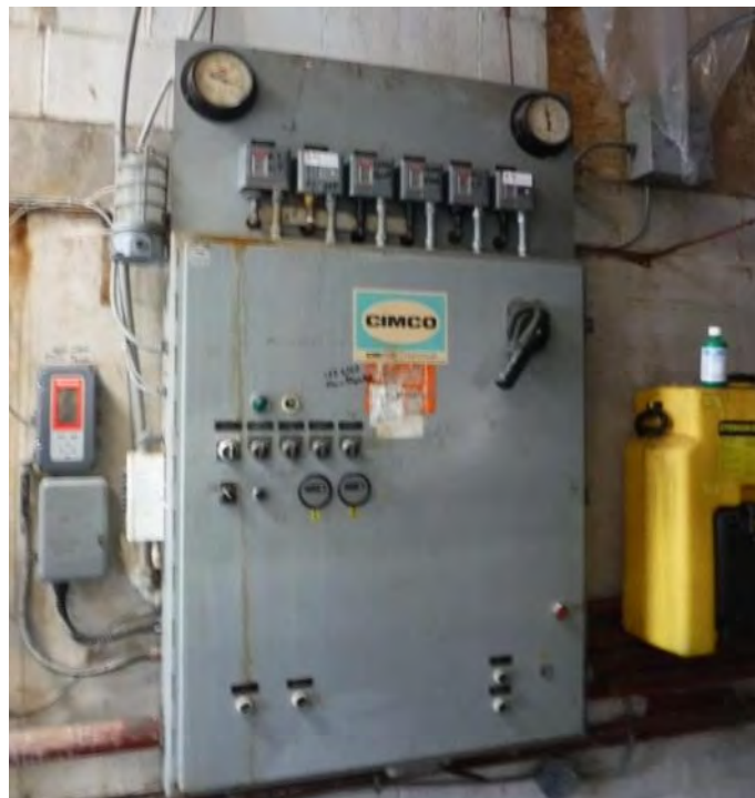
M6: Refrigeration Plant Control Panel
