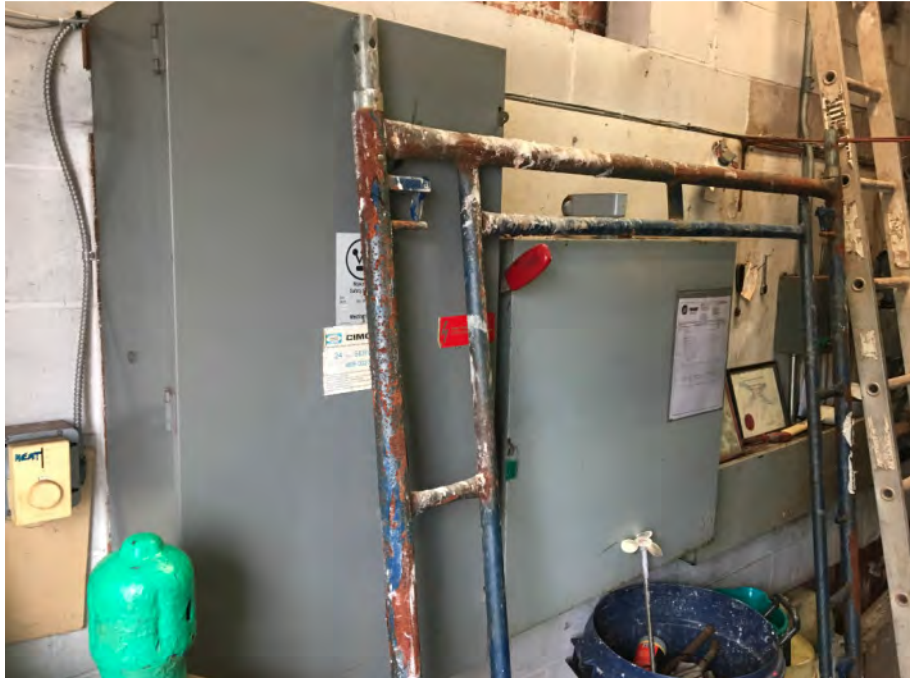
E1: Staging leaning on electrical equipment
