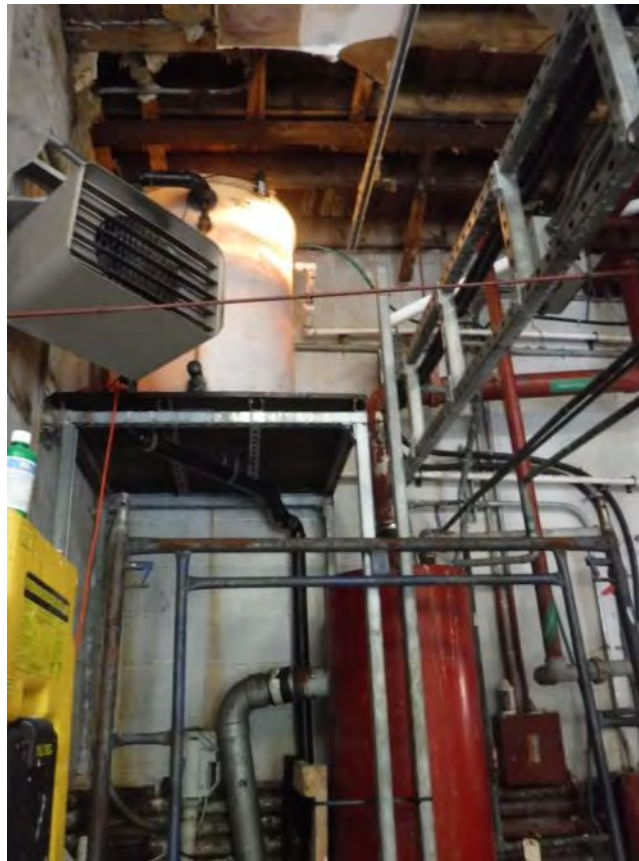
M7: Refrigeration Plant - Condenser water tank & mixing tank (note damage to ceiling)
