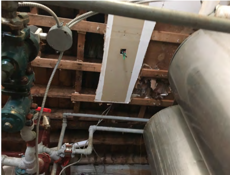
E5: Exposed wood ceiling in ice plant room near 600VAC equipment. One hour fire proof rated walls and ceiling is required.
