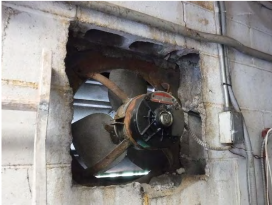
M10: Refrigeration Plant – Wall exhaust fan (require safety guard)
