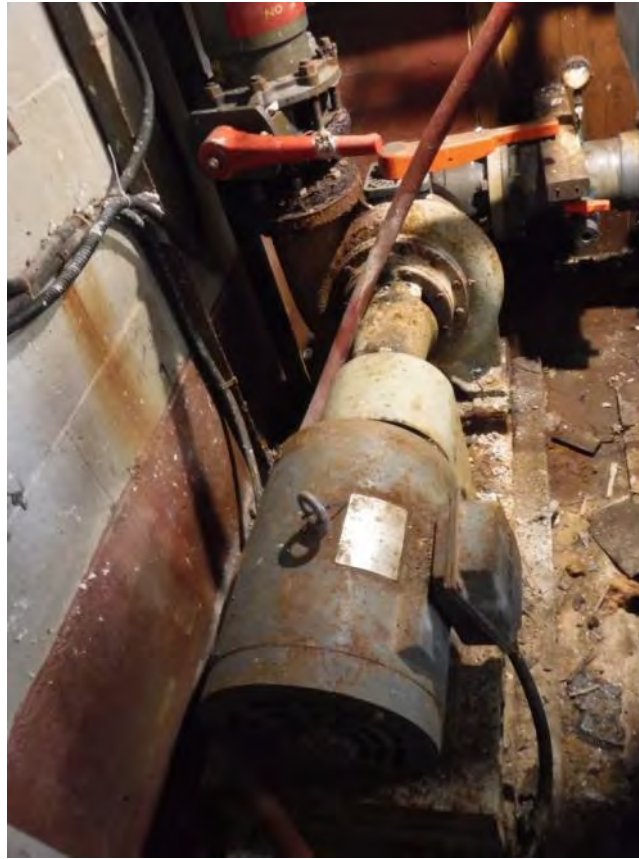
M8: Refrigeration Plant – Brine Pump #2 (installed 1985)
