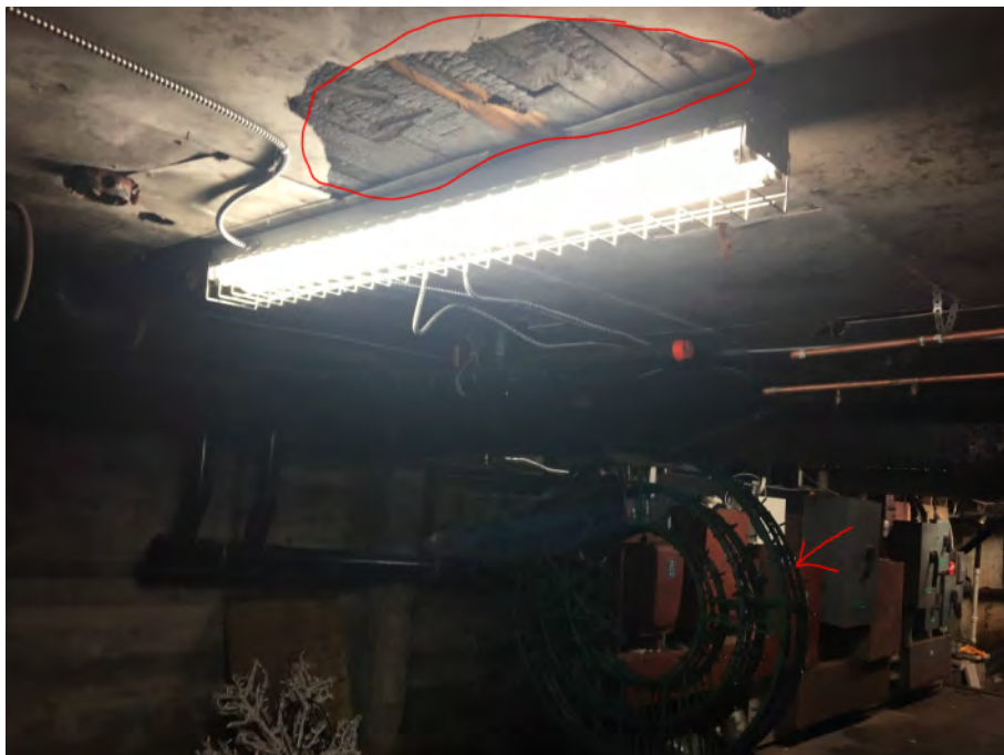
E8: One hour fire rating compromised by a previous fire
