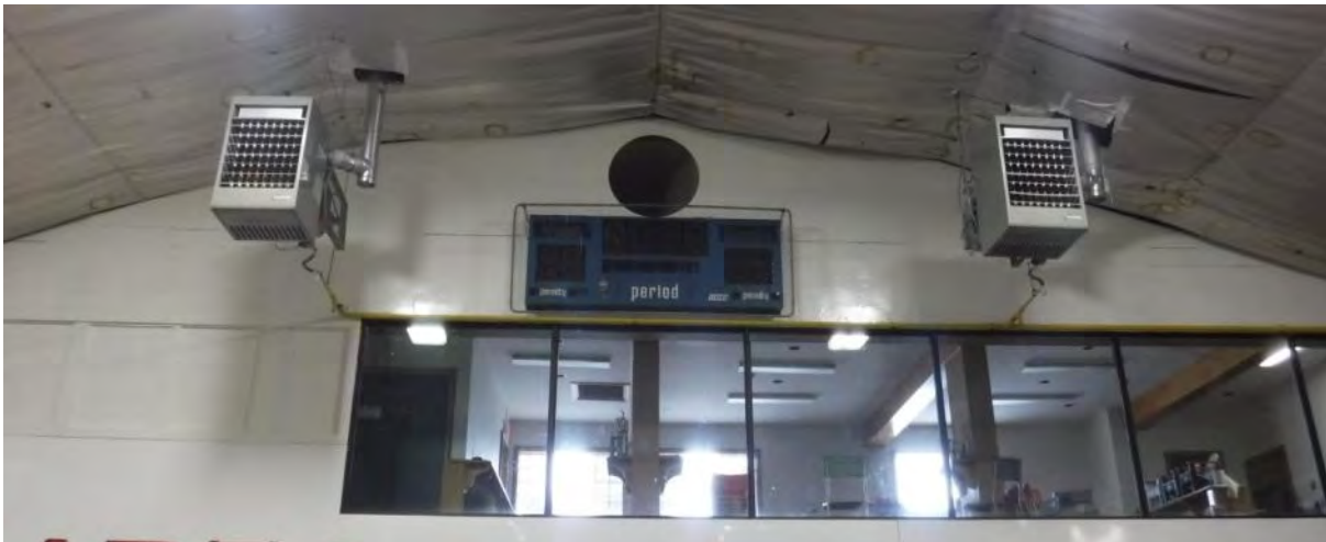
M15: Ice Surface Force Air Unit Heaters – Required for supplementary heat during non-Ice Season
