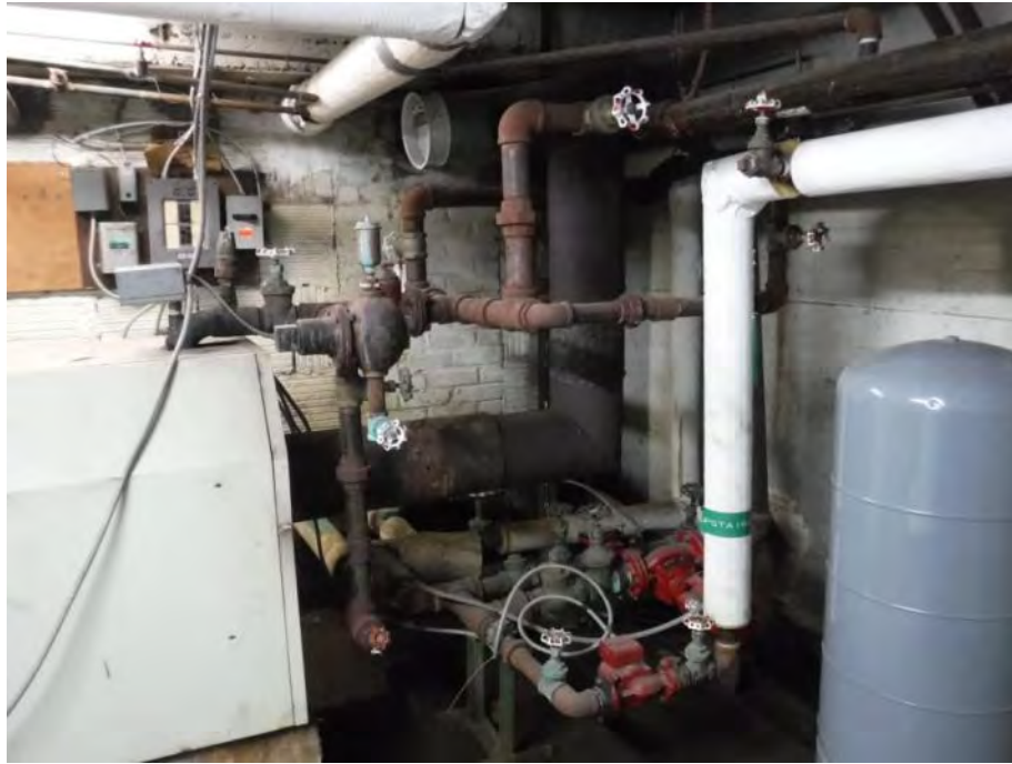
M12: Mechanical Room – Boiler System Breeching & Piping (breeching in poor condition)
