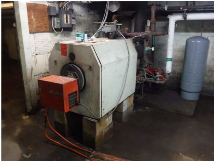
M11: Mechanical Room – Boiler System
