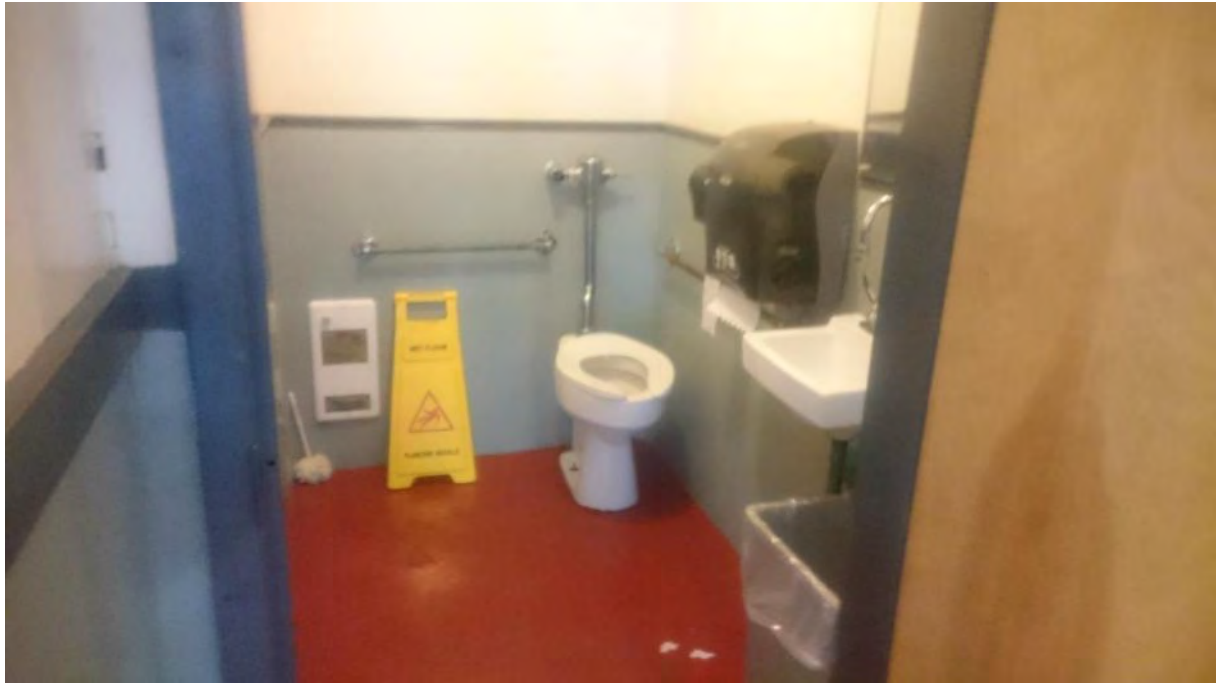
A9: Washroom off room #4. Door does not meet barrier-free requirements
