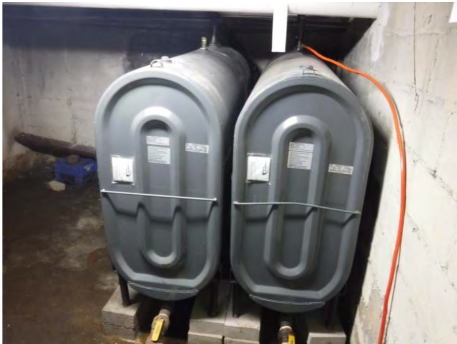
M13: Mechanical Room – Boiler System Fuel Tanks (tanks to be anchored to floor)
