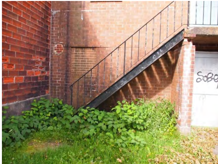
A2: Steel exit stair, uncontrolled plant growth
