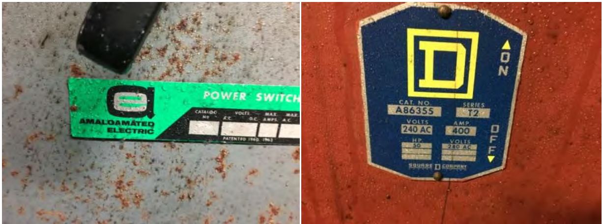
E11: Water condensing on metal Type 1 electrical enclosures due to lack of ventilation
