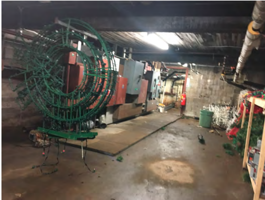
E7: Electrical Room used for storage
