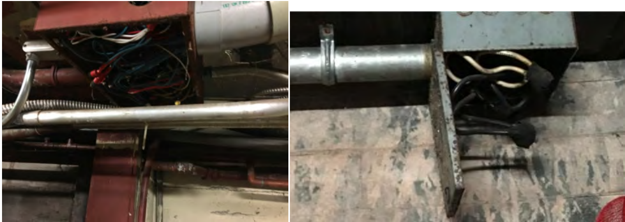
E9: Exposed wires, no cover on enclosures
