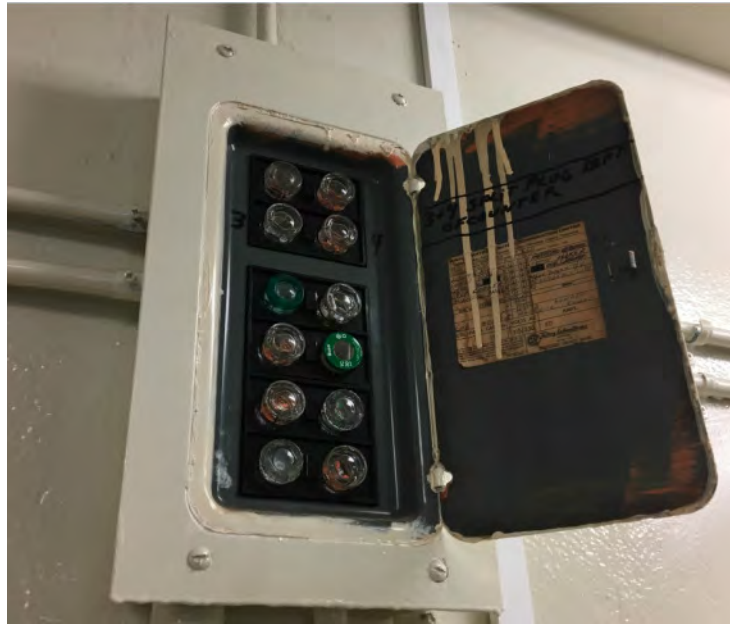
E16: Canteen fused panel. Consider replacing with a circuit breaker panel
