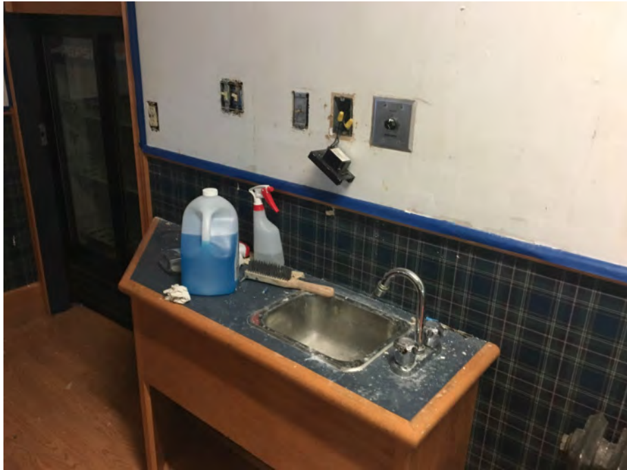
E18: Electrical switches and receptacles within 1 meter of a sink with no ground fault protection
