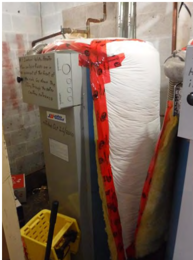
M17: Ice Resurfacing DHW heaters
