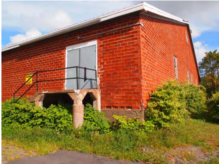
A3: Concrete exit stair, uncontrolled plant growth
