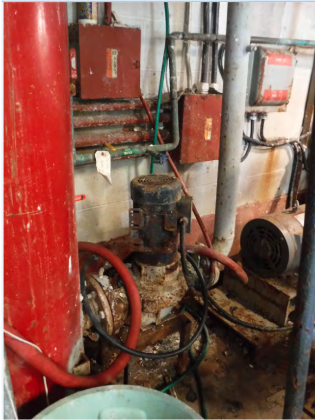
E3: Town Water line running on top of a 3-phase 600VAC manual Transfer Switch. Pipes obstruct one meter clearance in front of electrical equipment.
