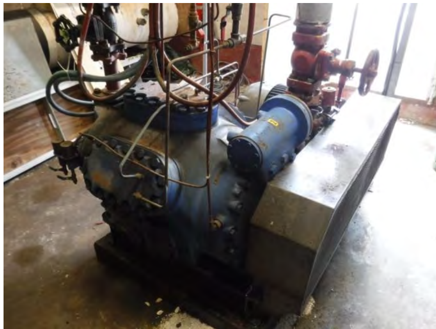
M4: Compressor #2 - J&E Hall 50 hp (installed in 1980)
