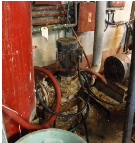
M8: Refrigeration Plant - Condenser Water Pump (installed in 2003)
