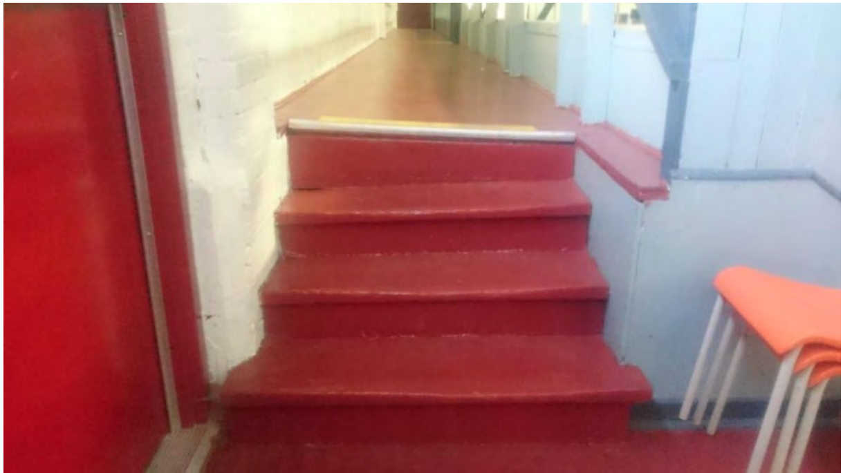
A7: Uneven stair and corridor behind stands
